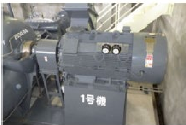
Figure 15. Energy Saving in Irrigation and Drainage Facilities (Upgrading to High-Efficiency Motors)
